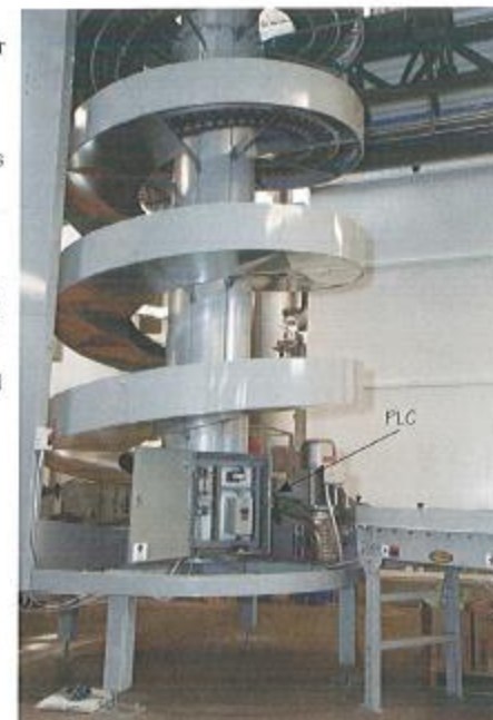
This PLC controls motors and sensors in an automated distribution facility, including this spiral conveyor system.
