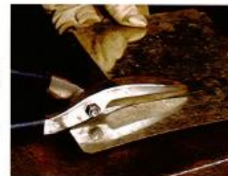
To cut a hole in sheet metal, first use a hollow punch to make a small hole inside the diameter of what will become the large hole. Then insert the tip of the snips into the punched hole. Cut in a circular pattern until the layout line is reached. Follow the layout line to complete the cut.
